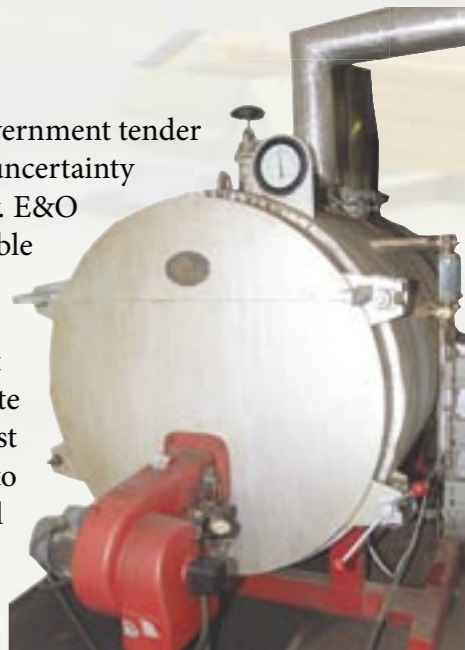
Back-up steam boiler
